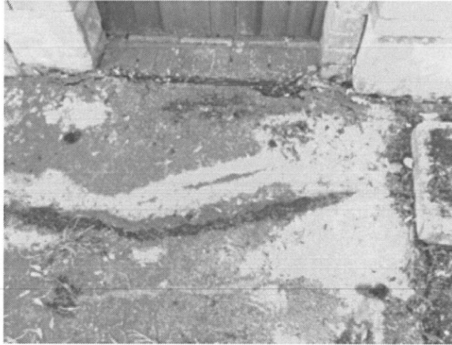
Damage to the driveway of Peterscourt from roots of Redwood tree (T4).
