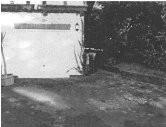
Damage to driveway and garage of 10, Plymouth Drive from roots of Redwood tree (T4).
